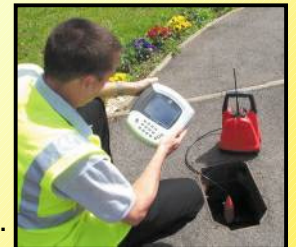
Step 2. Leak Pinpointing
