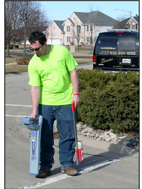
Locating buried utilities of all types is no problem for ATS Technicians
